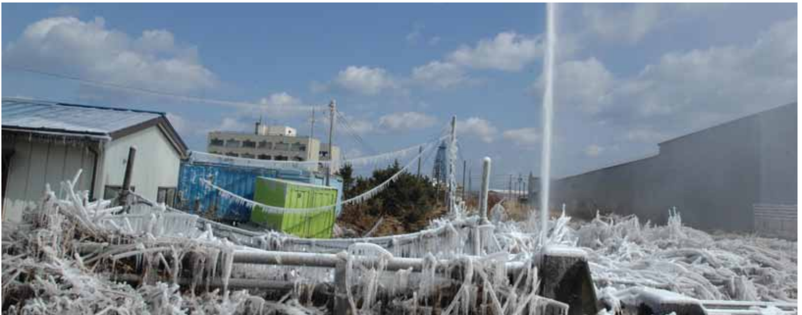
A water pipe spews water into the frosty morning air after being damaged by the tsunami in Japan. Unconventional systemic risks can trigger massive, instant, global upheaval, affecting climate, economy, health, environment and even the fabric of society itself
